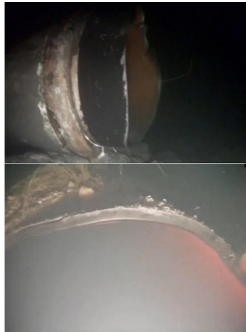
Figure 6. Destruction of the Nord Stream-1 pipeline section, initial inspection results Source: Nord Stream AG
